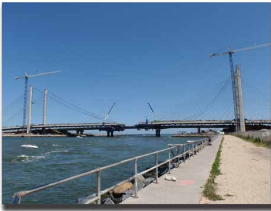
Construction of the new cable-stayed Indian River Inlet Bridge with the built-in fiber-optic sensor network is expected to be completed in spring 2012, with two lanes of traffic opening in December 2011. The existing bridge can be seen behind the new bridge. Photo courtesy of Gary Wenczel, University of Delaware.
